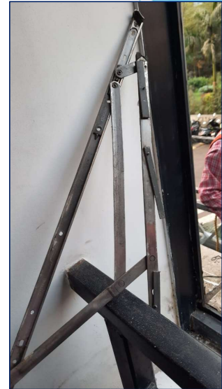
Broken Hinge Window 377
