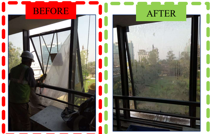
Window 59: Tied With Ropes due to Broken Hinges. Hinges replaced and Restrictor Arms installed.
