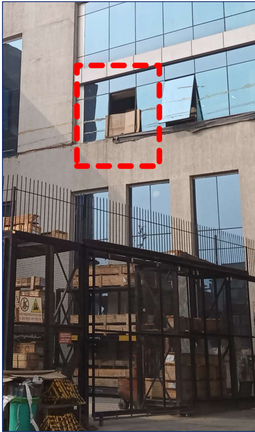
Broken Glass of Window 1507 ( Before )
